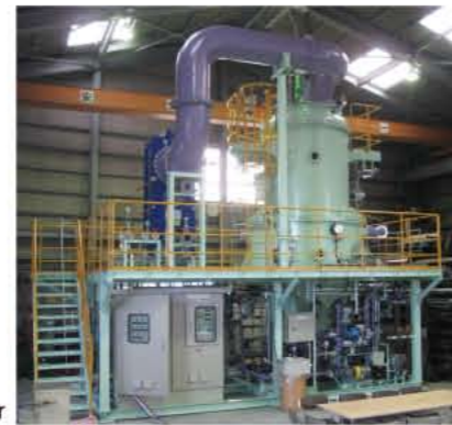
Ammonium chloride cooling crystallizer
